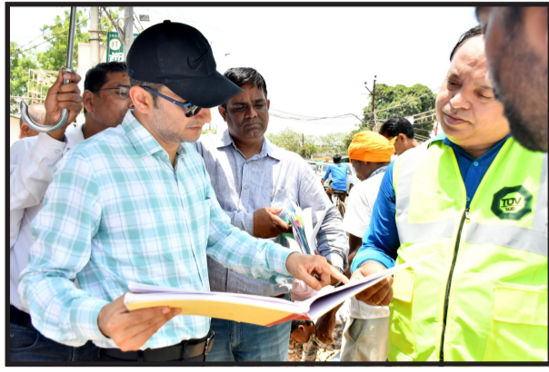
Road in Meerapur. During the inspection, the interlocking GSB thickness was found to be less at many places and the compaction was also found to be sub-
